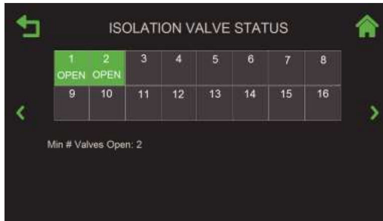
Figure 5.5: Isolation Valve Status Screen
