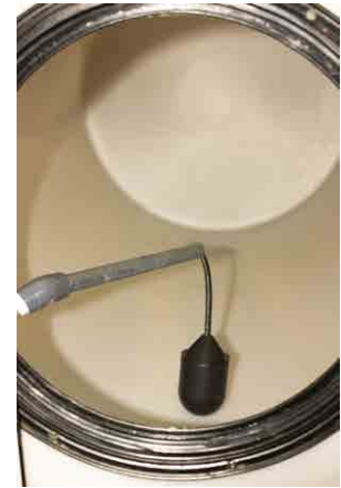
Pre Installed Float Switch
