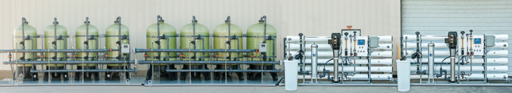
Custom system for distillery. Quad Micro-Z and Quad Carbon systems. Dual RO with a production of 110 gpm each operating at 380 volts, 3-phase, 50 Hz. with Antiscalant chemical feed.
